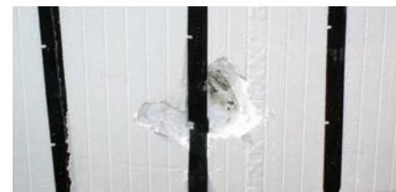
ARXX ICF wall - minimal damage
